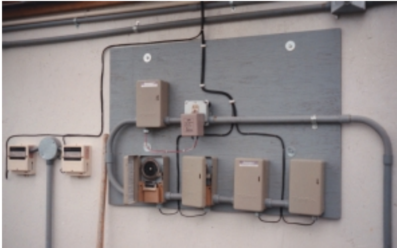
Picture 4. Control panel with timers.
